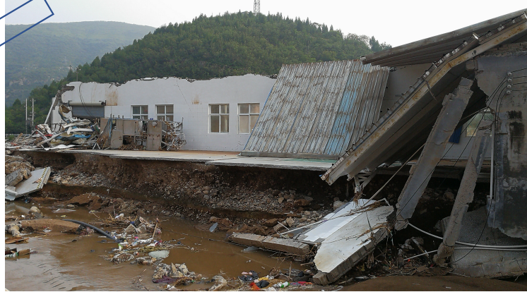
House destroyed by flash flood
