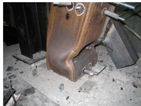
(c) local buckling of column
