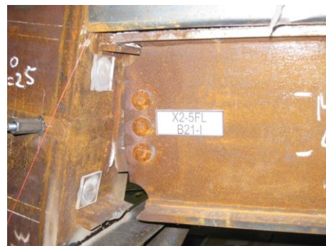
(b) fracture of beam end
