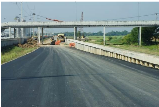
Figure 9 New dyke (finished grade) and elevated road north of Rojana IE (on the left)
