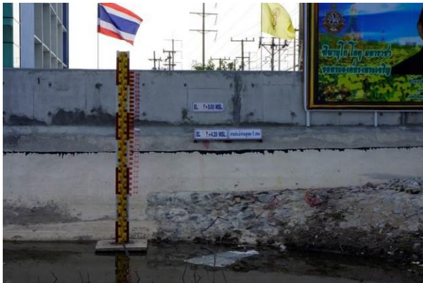
Figure 7 Upgraded dyke and flood wall in Bangpa-In IE (outer view) (Flood wall elevation pre 2011: +4.2m MSL; post 2011: +6m MSL)
