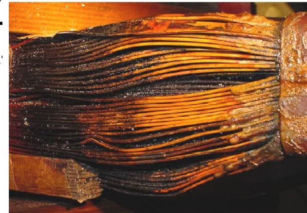
Station 3 Gen. Transformer 5 overheating
