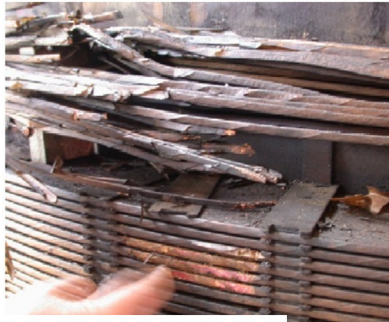
Station 4 Transformer 6 HV winding failure
