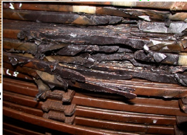
Station 3 Gen Transformer 4 damage
