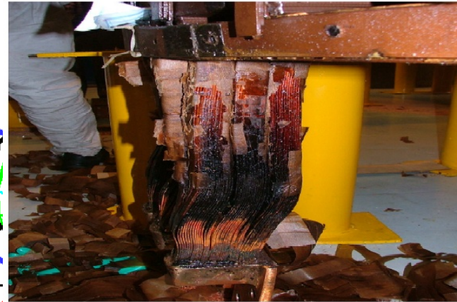
Station 3 Transformer 6 LV exit lead overheating
