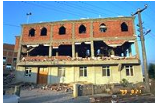
Figure 2. URM infill collapse
