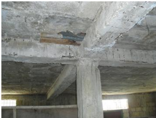
Figure 2. Beam With Exposed Reinforcement.
