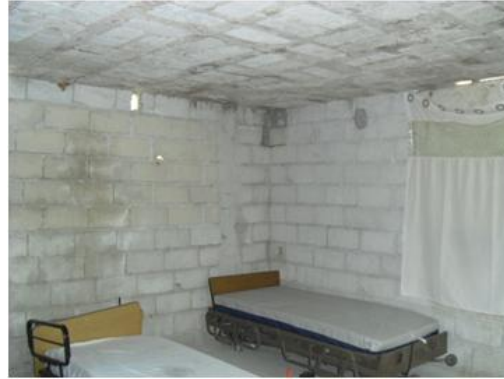
Figure 5. Poor Workmanship in Unreinforced HCB Wall
