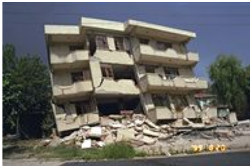
Figure 1. Soft story collapse in the 1999 earthquakes
