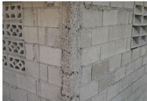
Figure 3. Poor Concrete Consolidation in Column
