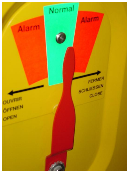
Figure 2: Example of tunnel equipment taken into account for alarming by TTC: lock of sliding doors closing off equipment and places of safety
