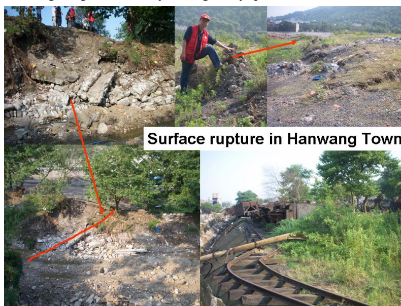
Fig.5 Surface ruptures and deformed Railway in Hanwang Town
