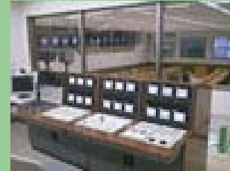
System operating room
