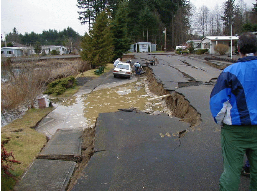
Figures 5 and 6: Photos of damage from the Nisqually Earthquake.
