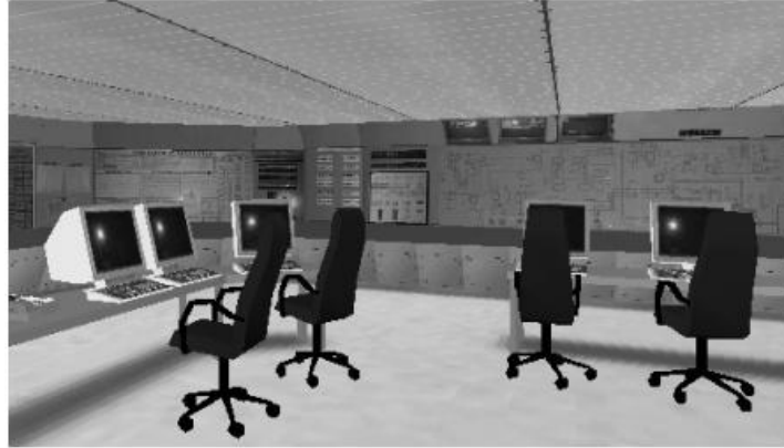
Figure 3 The offshore control room
